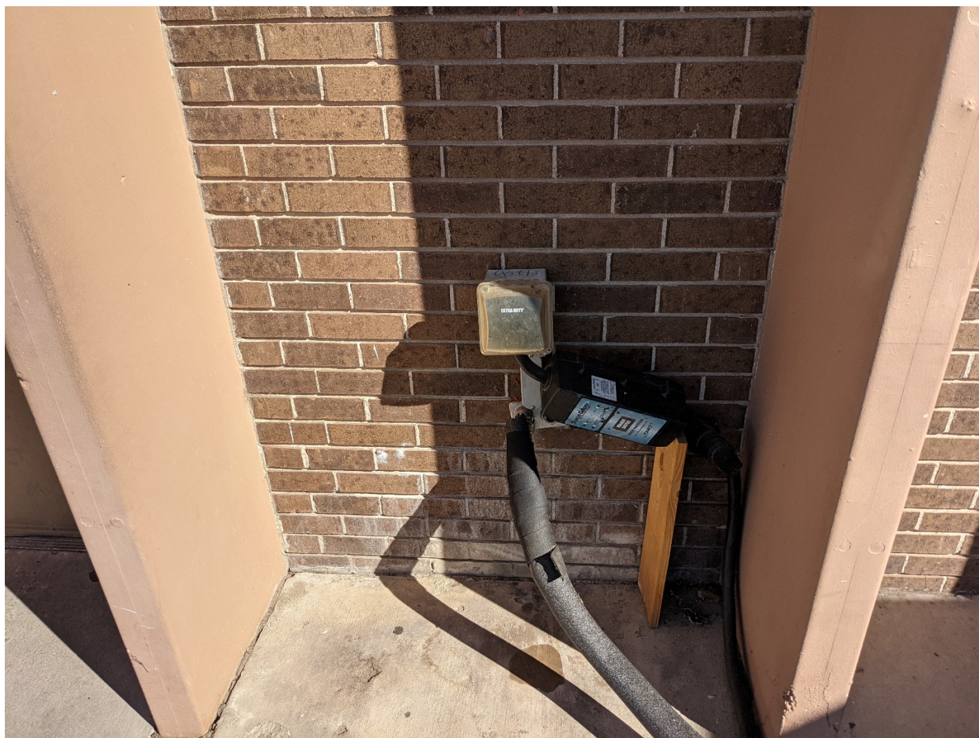
Code compliant electrical hook-up (September 16, 2021)
